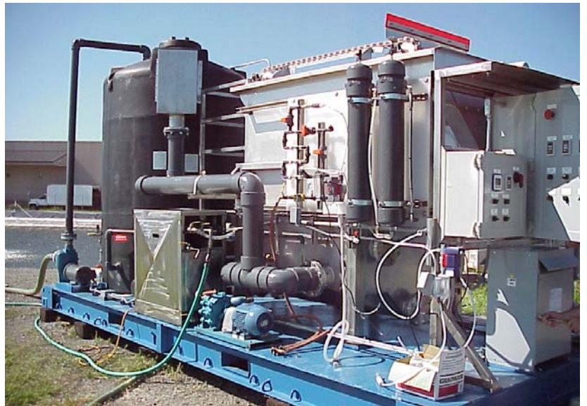
Skid Mounted SAF™ System Treating Wine Bottling Wastewater
