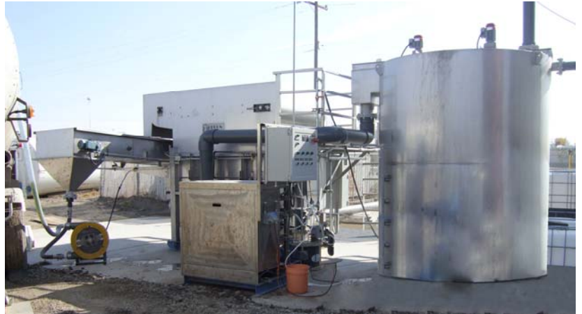
Complete SAF™ System Treating Food Processing Wastewater
